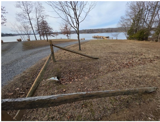
Gravel drive and split rail fence — fence rail appears loose/leaning (Items #4, #7)
