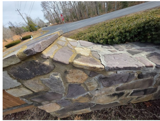
Monument cap — visible cracked/failing mortar joint (Item #1)
