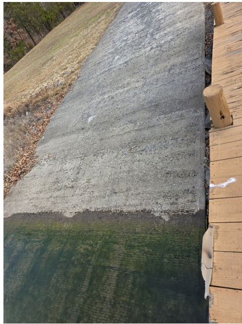
Concrete boat ramp at the waterline — algae/staining visible on the lower ramp surface (Item #19)
