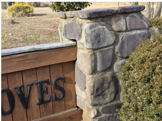
Entrance monument cap — cracked/spalled cap stone, consistent with the overdue repointing item (Item #1)
