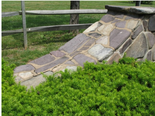
View of west side entrance monument sloping cap failing mortar
