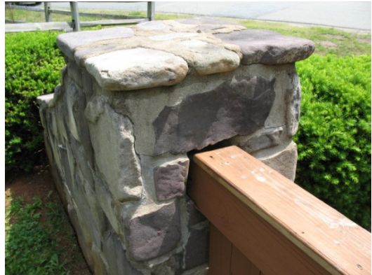
View of west side entrance monument failing mortar below cap
