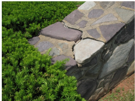
View of east side entrance monument sloping cap failing mortar
