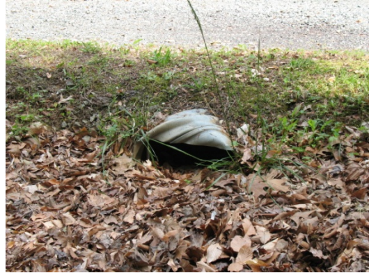
View of culvert pipe inlet - leaves should be removed
